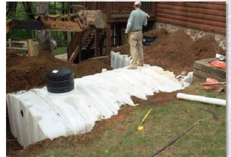
Tank kept under house; filter prior to system entrance
