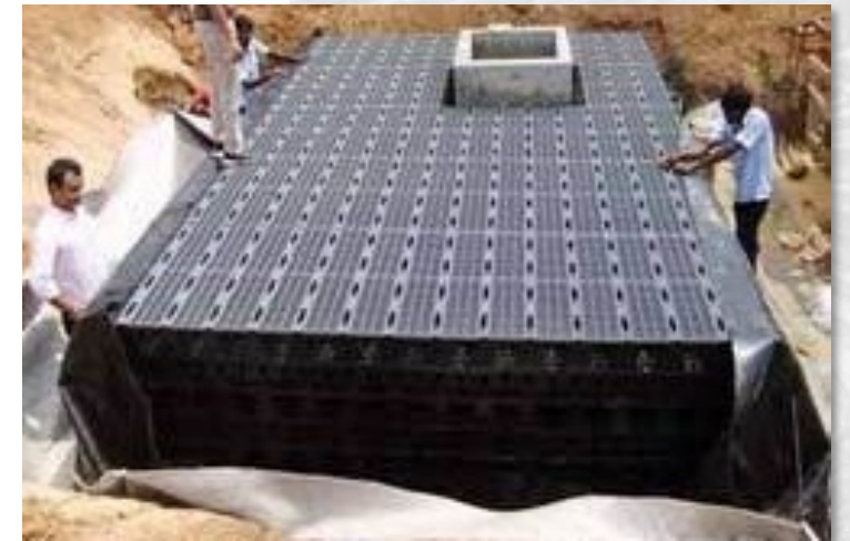
Technical rainwater harvesting in 'rigola' system
