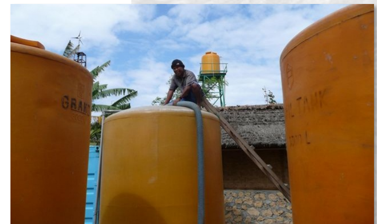
Aboveground storage tanks for transported water
