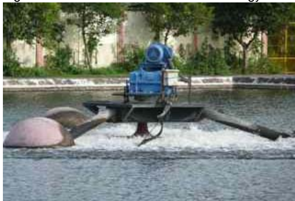
Figure 6.12: Facultative Aerated Pond – Yogyakarta
