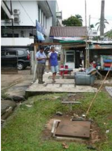
Figure 6.20: Pumping station and tanker discharge chamber at Indraprasta
