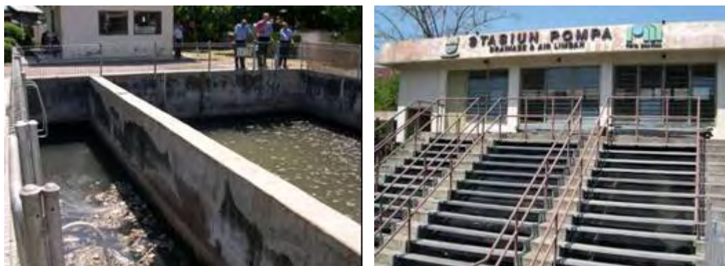
Photo by: Oni Hartono Date: October,06 '05 Location: Pump station Wastewater Ade Irma - Cirebon Remarks: Equalization tank and pump station.
