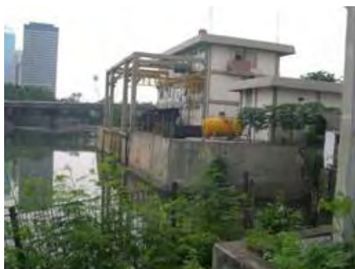
Photo by: Edzard Ruehe Date: October,3 '05 Location: Jl. Setiabudi - Jakarta Remarks: Pumping house to discharge wastewater from Waduk Setiabudi to Banjir Kanal River
