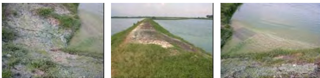
Photo by: Oni Hartono Date: October,10 '05 Location: WWTP 'Bojongsoang' - Bandung Remarks: Algae (green color) found in Facultative Pond. Very strong smell.
