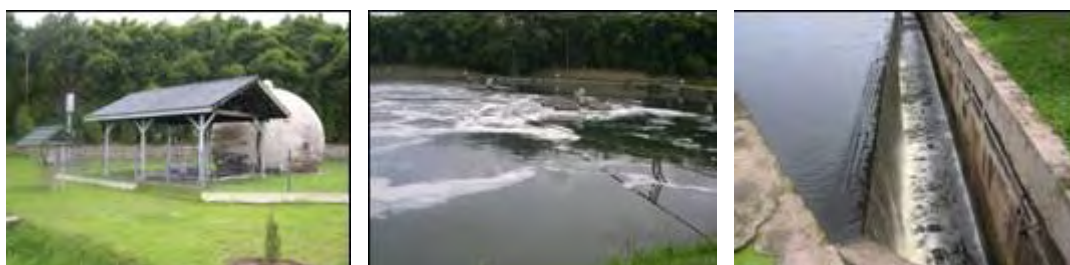
Photo by: Edzard Ruehe Date: November,29 '05 Location: WWTP Pulau Brayan Bengkel (Cemara) – Medan Remarks: (From left): Gas storage from UASB ; Aerated Pond ; Outlet (overflow) to Kera river
