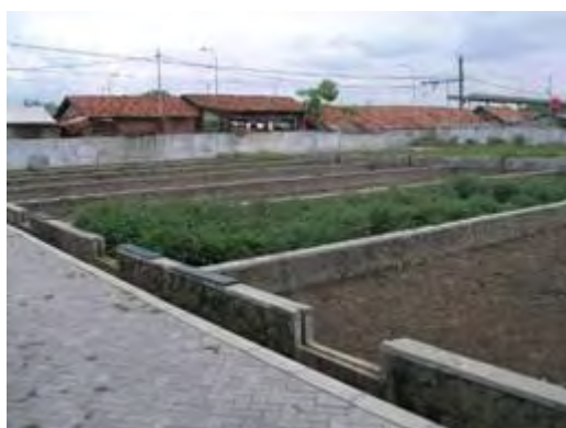
Photo by: Edzard Ruehe Date: October, 19 '05 Location: WWTP 'Tanah Tinggi' – Kota Tangerang Remarks: Sludge Drying Bed.
