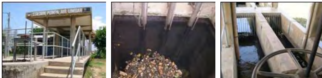
Photo by: Edzard Ruehe Date: October,06 '05 Location: WWTP Kesenden – Cirebon Remarks: (Centre) equalization tank and submersible pumps. (Right) bar screen with gate water.
