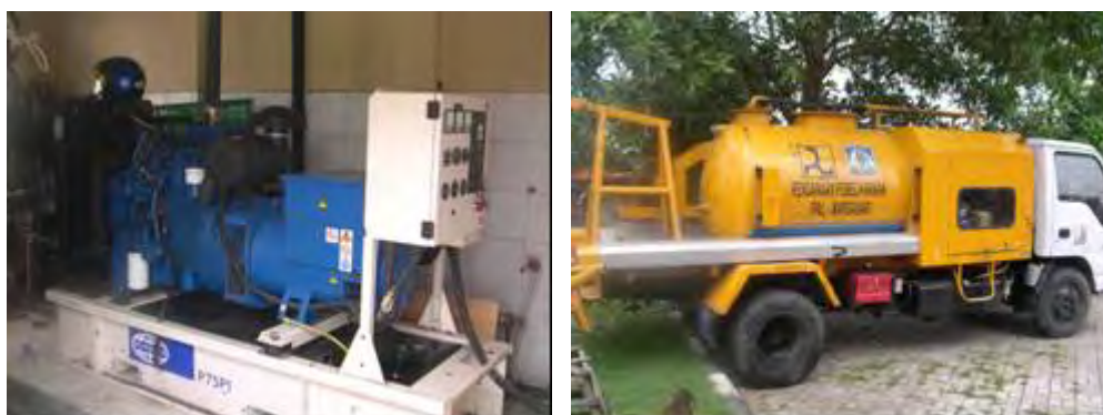
Photo by: Edzard Ruehe Date: November, 14 '05 Location: WWTP Margasari - Balikpapan Remarks: Left picture: genset (in WWTP Margasari) Right picture: truck for maintenance of sewerage pipe (flushing).
