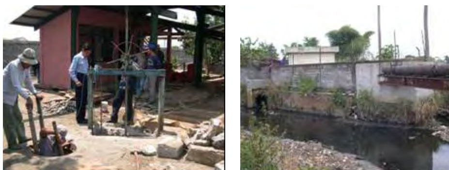
Photo by: Edzard Ruehe Date: October,10 '05 Location: Station pump – Cijawura - Bandung Remarks: (left picture): Pumps unit in Cijawura, pumping wastewater to WWTP Bojongsoang. Pump station still under rehabilitation. (right picture): Outlet from pumps (see on the right) to WWTP Bojongsoang has a hole (see on the left) by-passing wastewater direct to the river (Cidurian River).
