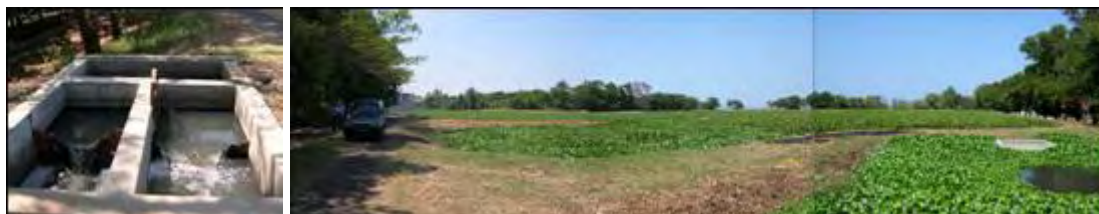
Photo by: Edzard Ruehe Date: October,06 '05 Location: WWTP Ade Irma - Cirebon Remarks: (from left) inlet unit ; aerated pond (with eucalyptus plants).
