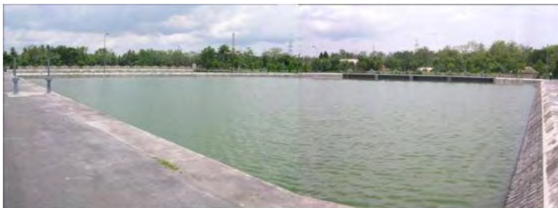
Photo by: Oni Hartono Date: October,25 '05 Location: WWTP Sewon – Bantul - Yogyakarta Remarks: Maturation Pond, outlet with weir.
