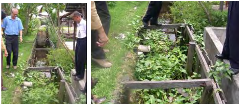
Photo by: Oni Hartono Date: November, 14 '05 Location: WWTP Margasari - Balikpapan Remarks: Outlet from WWTP Margasari (with pipe PVC Ø 150mm), water goes to Pandan Arum river.
