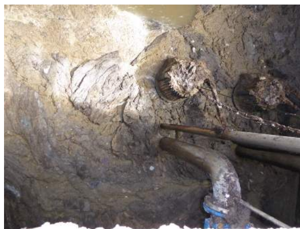
Figure 5: Pump sump with scum layer
