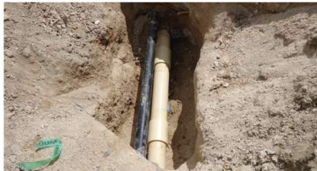
Figure 14: Pipes in one trench, too close to each other (Source: Dorsch, 2015)
