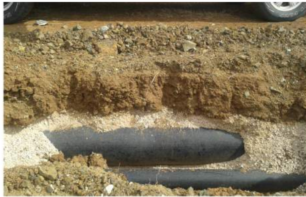
Figure 13: Lack of distance between pipes in trench (Source: Dorsch, 2015)
