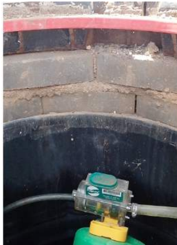
Figure 12: Masonry on top of vacuum pit that could lead to infiltration of storm water (Source: Dorsch, 2015)
