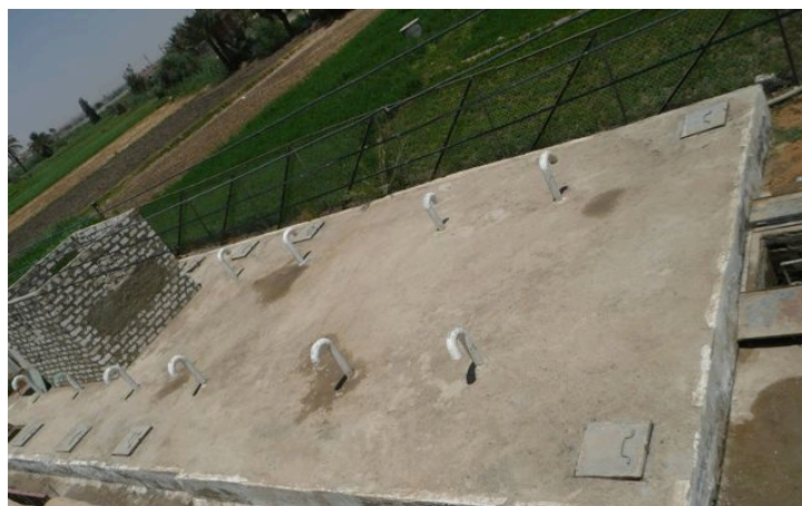
Figure 33: Settling tank and Anaerobic Upflow Filter
