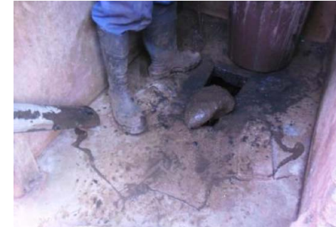
Figure 74: The sludge is often so thick and solid that rocks like this are suspended and are loosened during the fluidising process.
