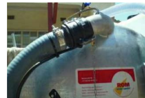
Figure 21: The plastic clamps were not durable and we experienced air leaks.
