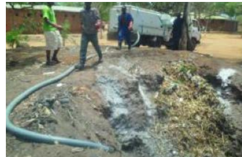
Figure 30: Increased length of discharge pipe – to make it safer and easier to discharge into a sewage disposal or pit.
