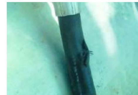
Figure 37: The pressure hose burst – it was seen that the pressure regulator was mistakenly set too high.
