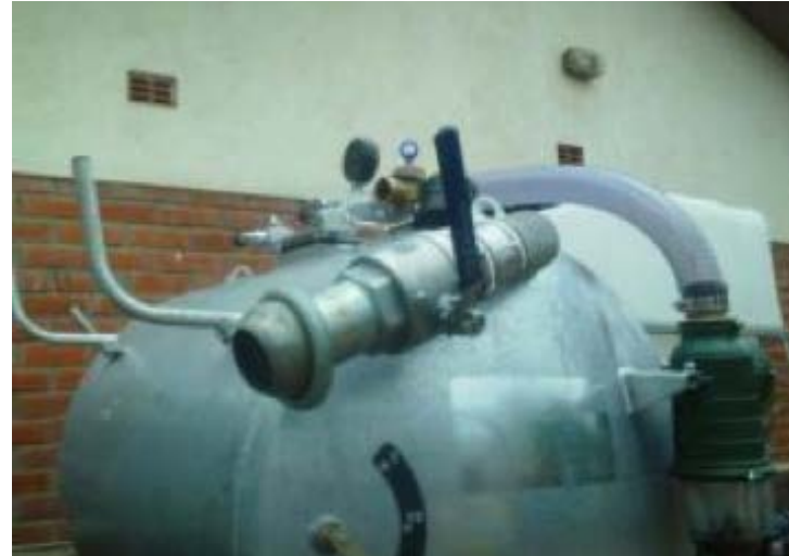
Figure 22: We changed to a metal and have observed they are more durable and have no air leaks. We changed the suction valve from plastic to metal. It is easier for the truck side operator to control the suction valve. The elbow somehow restricts the flow of the thick sludge.
