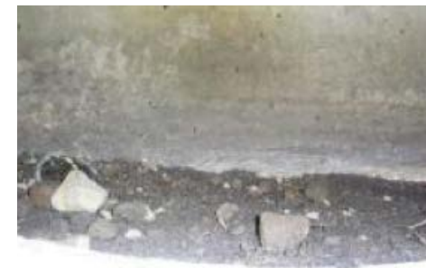
Figure 44: One can see stones, charcoal and other debris through the inspection cover. The tank will now be easier to clean and service in case of can blockages or sticking full / empty gauge.
