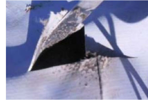
Figure 84: We opened the outer layer puncture in order to repair the inner layer, but found that sludge had leaked from the bladder in between the layers. This meant we could not access the inner layer for repairs. We just repaired the outer layer.
