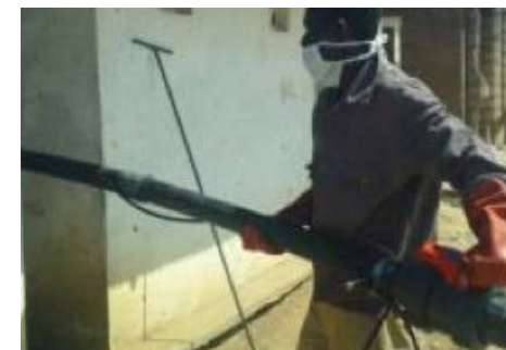
Figure 18: Due to the small doors, the lance and the suction pipe had to be assembled inside the toilet.
