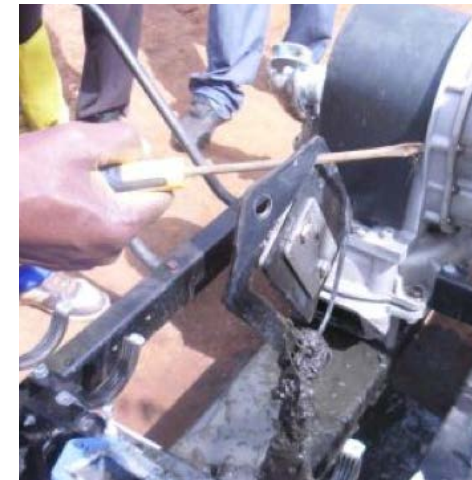
Figure 67: Suction port is not sealed due to a small piece of cloth.
