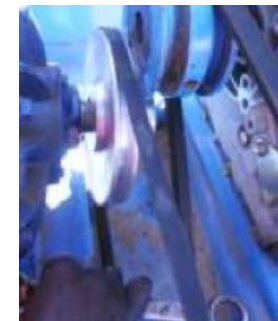
Figure 58: The pulley fitted on the machine. Note that the pulleys and belts are unprotected.
