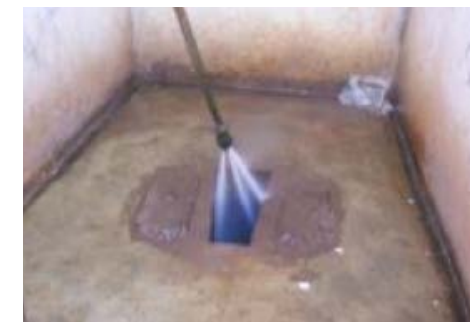
Figure 2: The water jet is also essential for cleaning the toilet slab and the desludging equipment.
