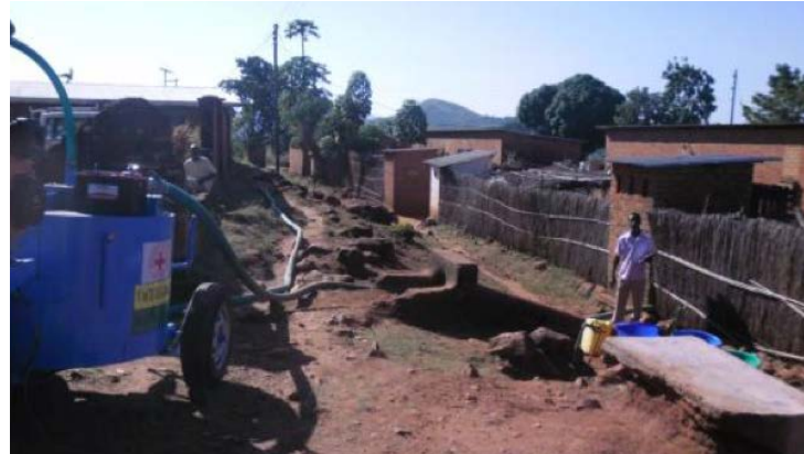
Figure 72: With fluidising the Vacutug was able to access and empty hard toilet sludge from a distance of 30m and an elevation of 2m. The Karcher fluidiser is next to the toilet (white building in the background). Otherwise the toilet would have been inaccessible.
