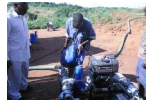
Figure 63: The pump requires priming with water.
