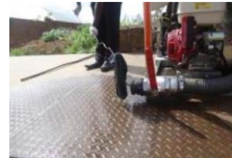
Figure 33: Some of the blockages were easily removed using a wire hook: in this case a pair of panties were removed from the discharge side.
