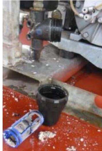
Figure 38: The filter body housing and the filter dismantled. The gauze of the filter has been perforated and there was a lot of sediment found in the filter housing.
