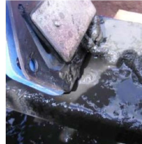
Figure 66: Suction port is not sealed due to a small piece of cloth.
