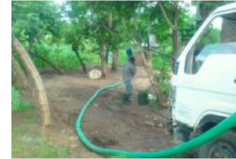
Figure 40: The Toilet is 30 m away – and inaccessible by the truck. Pressure hose to the right of the suction pipe.
