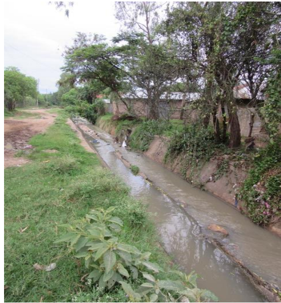
Figure 5: Lined Storm Water Drain Used as Open Sewer in Manyatta
