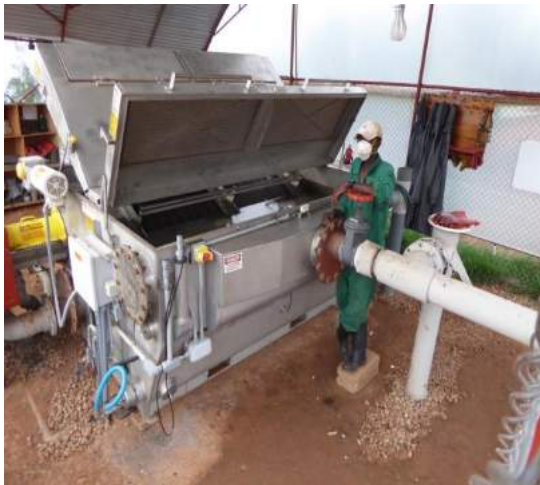
Figure 56: Micro screen type mechanical dewatering, Pivotworks Kigali (January 2016)
