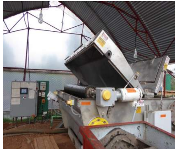
Figure 57: Belt filter press (Pivotworks, Kigali, 2016)
