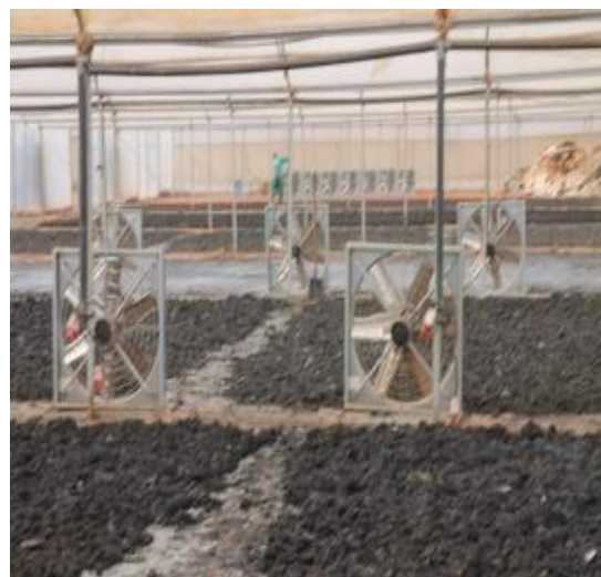
Figure 12: Drying Faecal Sludge in Greenhouse by Pivotworks
