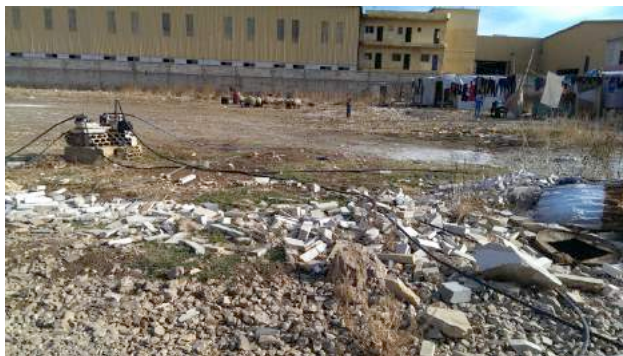
Figure 11: ITS T'nayel 005, Lebanon: flooded areas in winter, left water bore hole, right grey water infiltration pit
