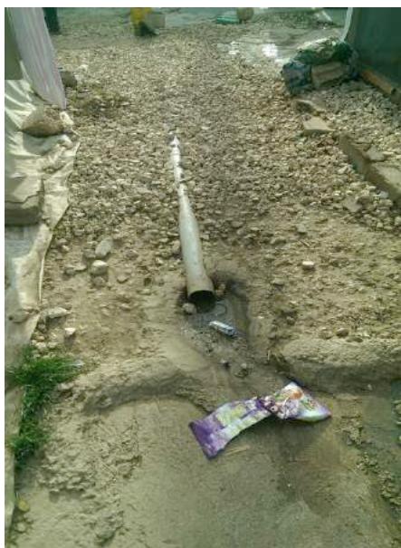
Figure 12: ITS Zahle Mualqa 019 grey water connected to storm water drain
