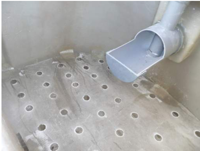
Figure 67: Interior Anaerobic Upflow Filter Tank
